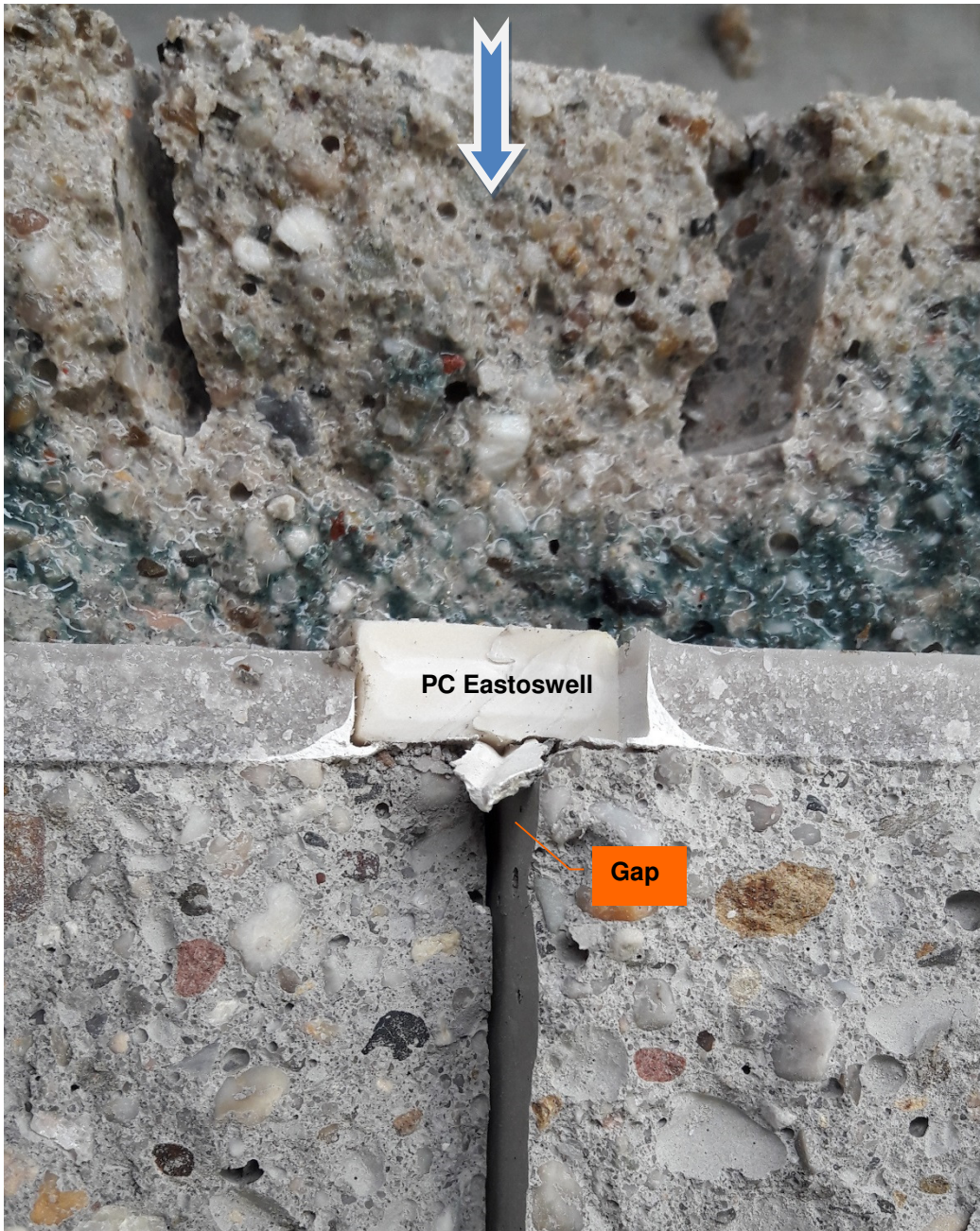
Photo 4. Configuration C, Detail of PC Elastowell, no leakage visible
